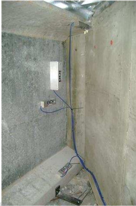
Figure A-5 Surface-mounted sensors (vibrating wire gages and tiltmeters) at girder ends.
