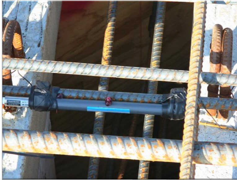
Figure A-3 Strandmeters installed on reinforcing bars in deck over continuity diaphragm.
