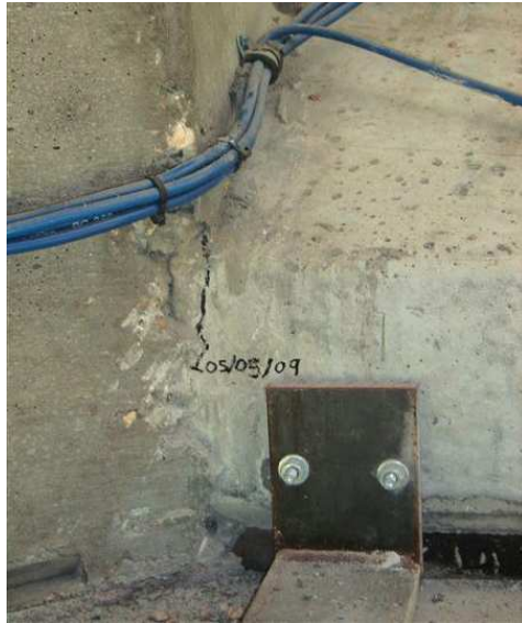
Figure 32 Observed crack at bottom flange of Girder G3 – Span 24.
