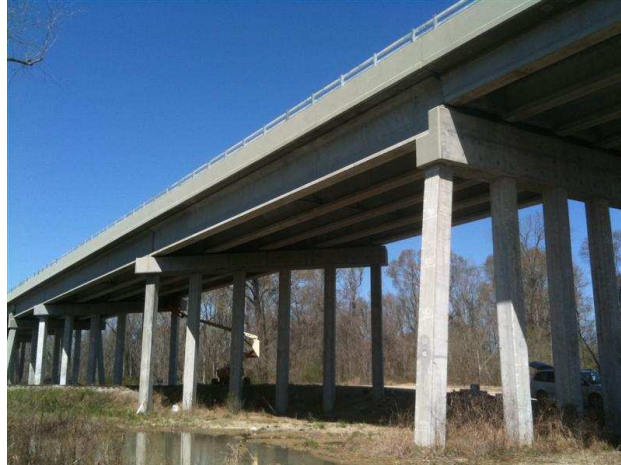
Figure 29 Sunlight hitting the bottom flange of G5 while the top flange is shaded by the overhang.
