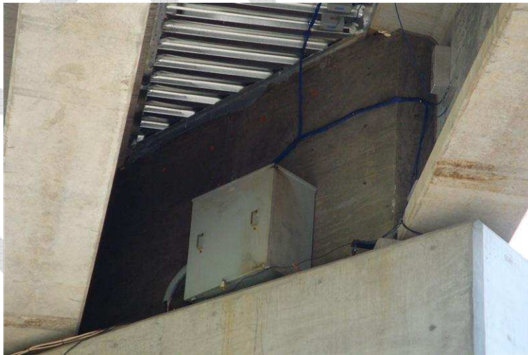
Figure A-12 Datalogger location in the complete system at bridge site. (Bent 24)
