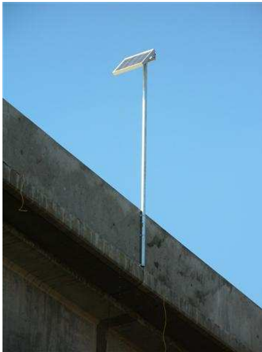
Figure A-9 Solar panel powering the monitoring system.
