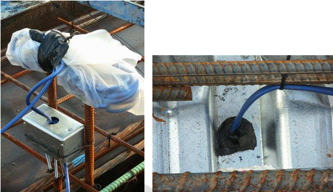
Figure A-7 Protection of wiring for embedded sensors prior to concrete casting.
