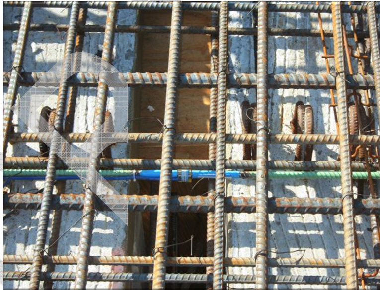
Figure A-4 Sisterbars installed next to reinforcing bars in deck over continuity diaphragm.
