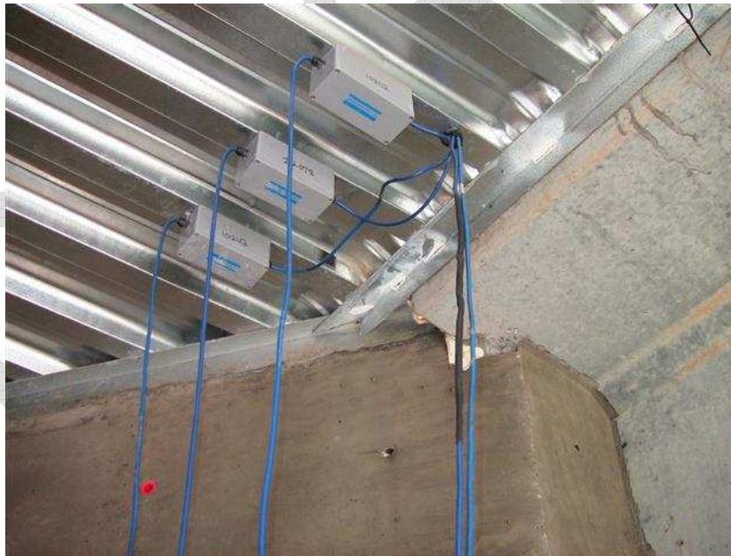
Figure A-8 Surge protectors installed on one of every two embedded sensors at the same location.
