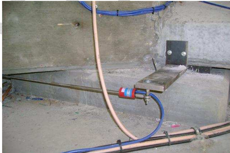
Figure A-6 Gap meter installed on brackets connected to girder ends at continuity diaphragm.
