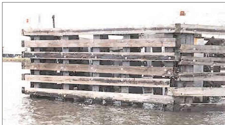
A typical Louisiana pier fender
