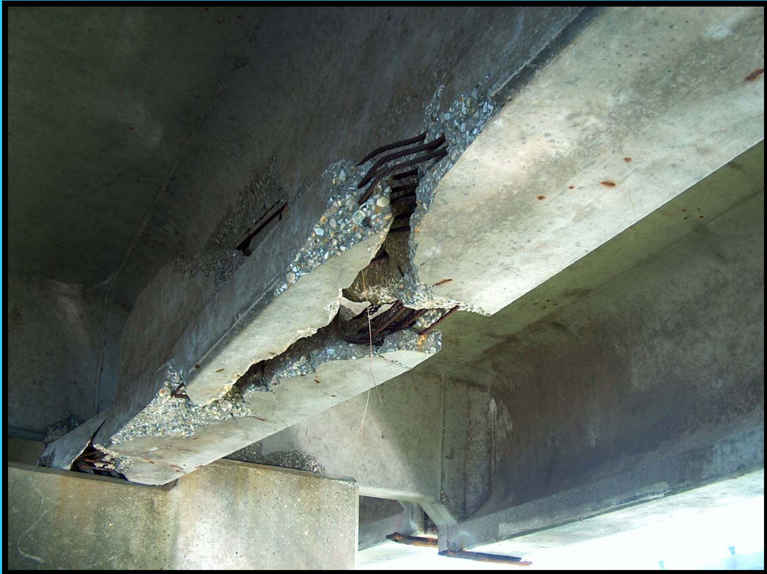
Broken girder end with exposed strands
