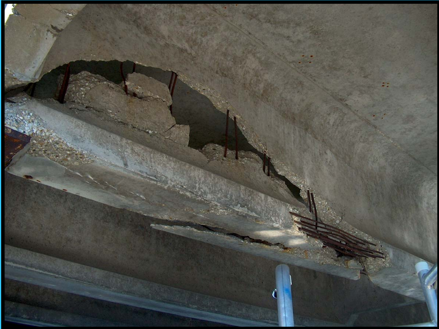
Broken girder end with exposed strands (bearing on left)
