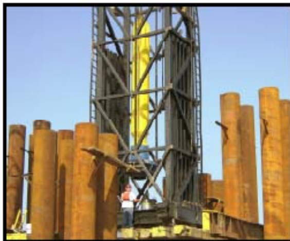
A member of the construction team inspects the pressure chamber during statnamic testing.
