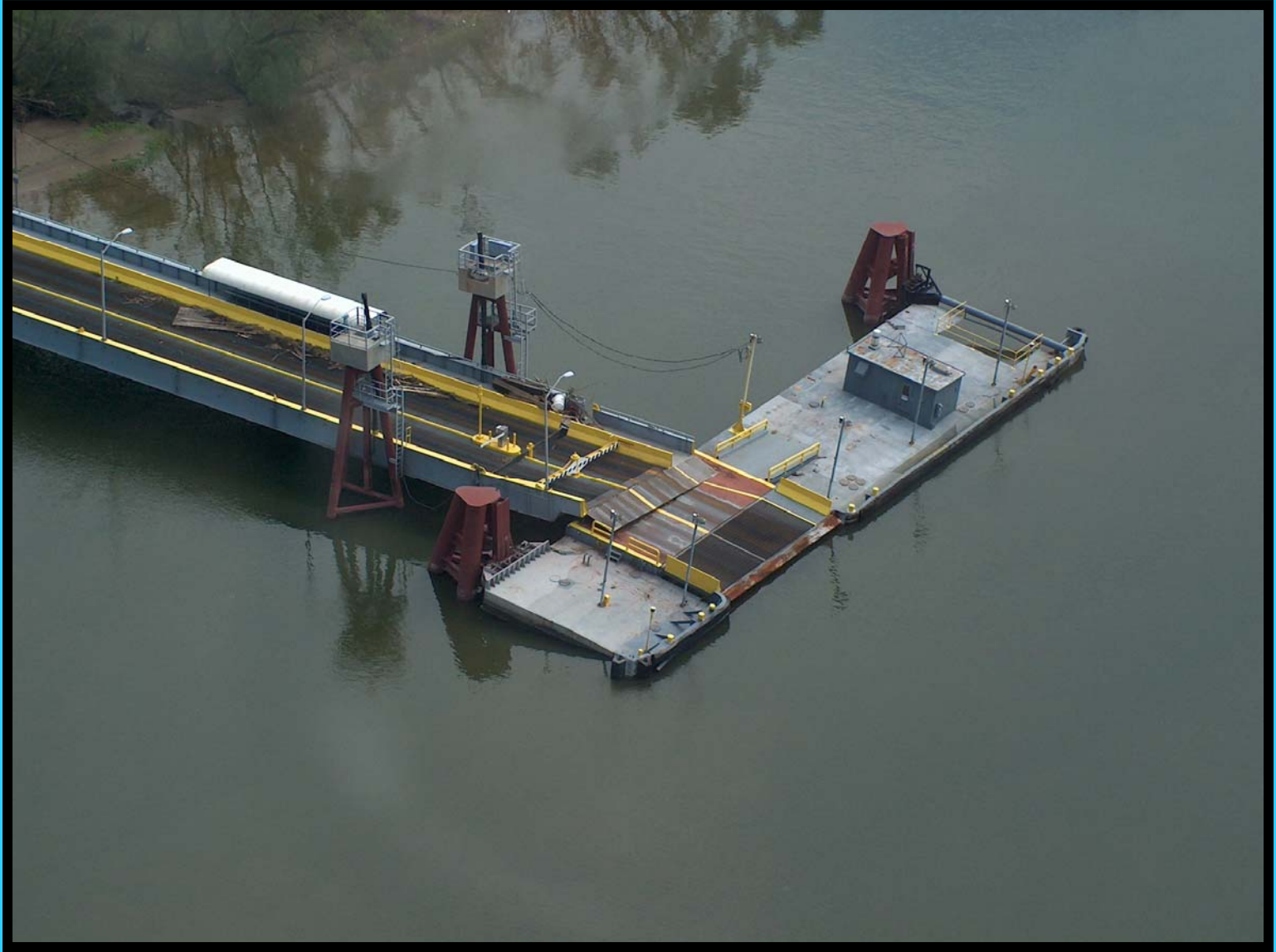
DAMAGED CRESCENT CITY CONNECTION FERRY LANDING
