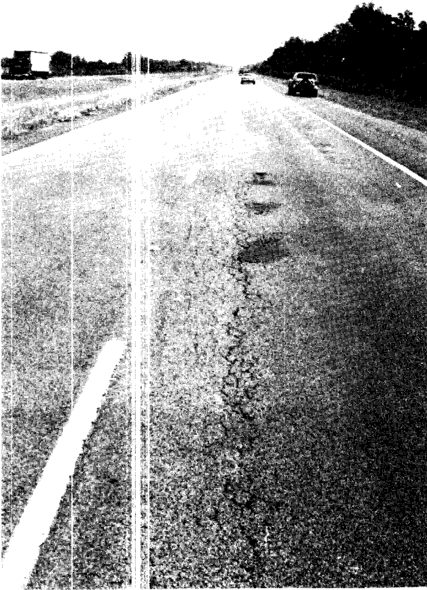
Wheelpath Cracking and Patching Figure 6
