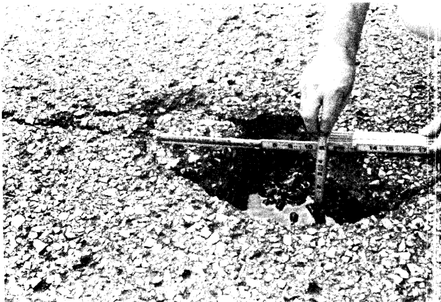
Pothole Where Wearing and Binder Course Have Broken Out Figure 13
