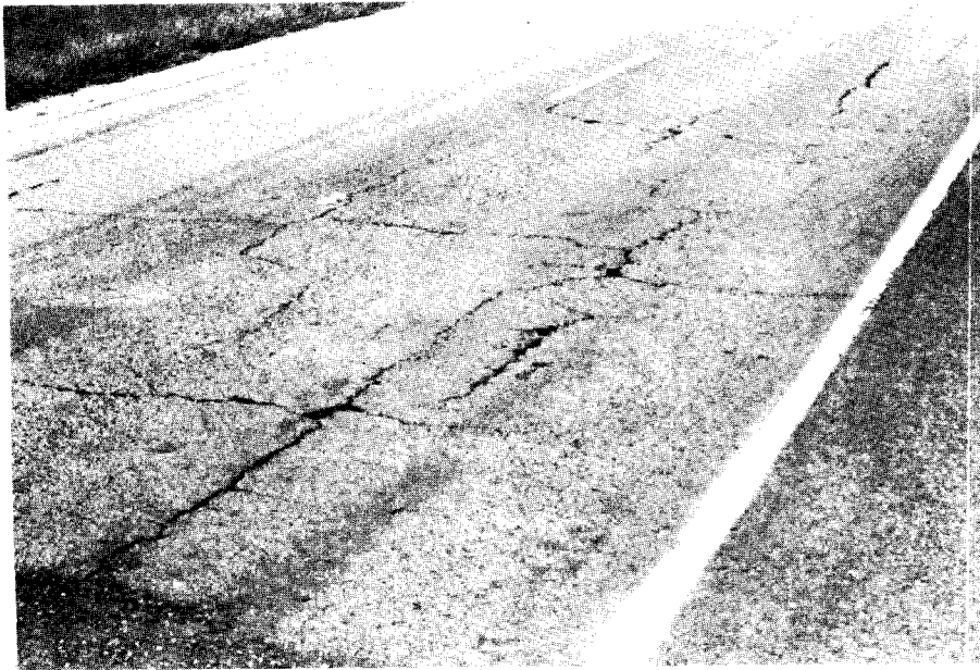
Potholes Develop Where Cracks Intersect Figure 12
