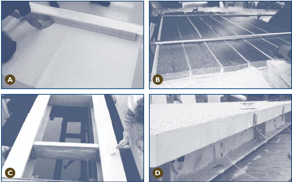
Figure 1 Researchers fasten bridge deck units with GFRP sheet and balsa wood beams
