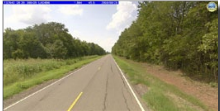
LA 494 pavement distress (longitudinal cracks)
