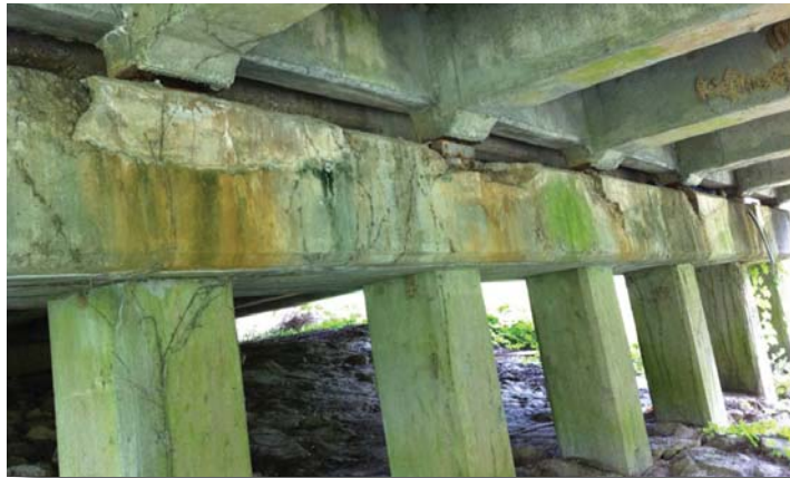
Figure 1 Spalling of concrete at bearing locations
