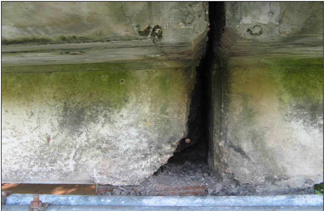
Figure 16 Damaged Beam Bearing @ Pier 4.
