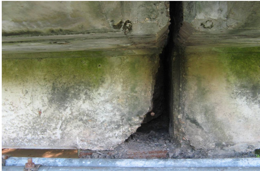
Figure 26 Damaged beam bearing at Pier 4
