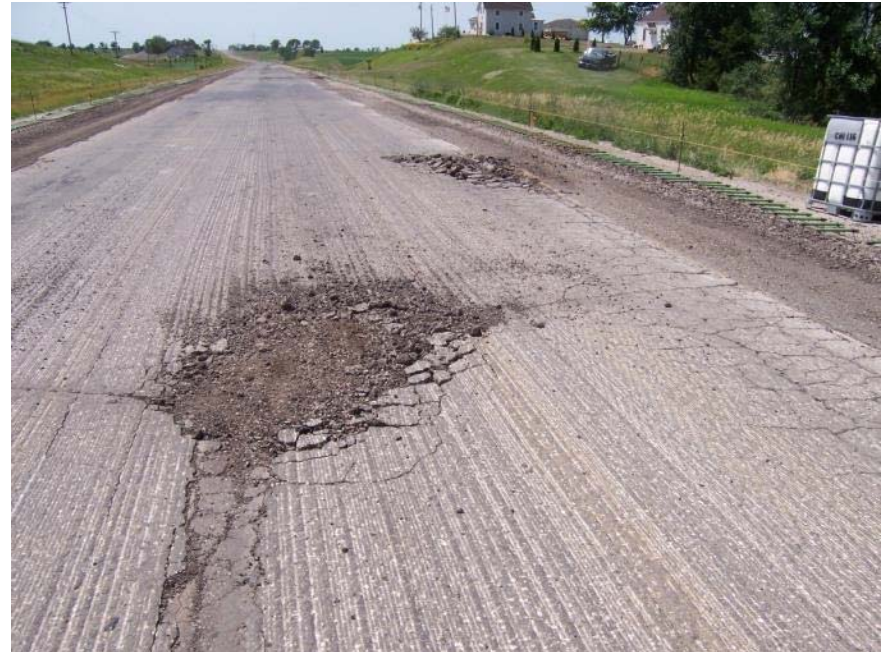
Excessive milling of existing asphalt
