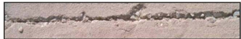
c) Unacceptable raveling—sawed too early
