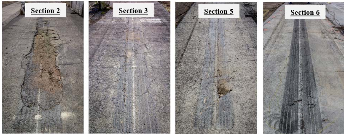
Figure 28 RCC pavement condition at the end of testing
