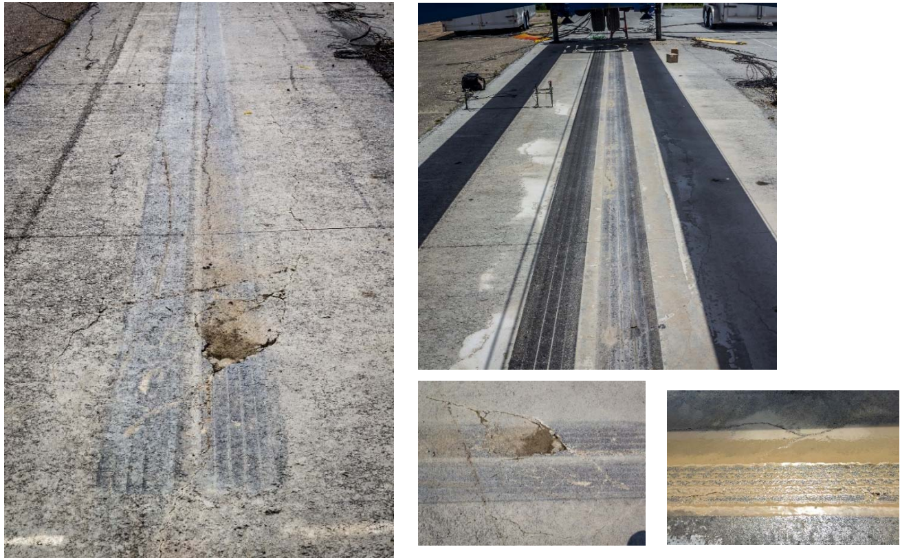
Figure 43 Distresses observed on Section 5 (6+8.5RCC)
