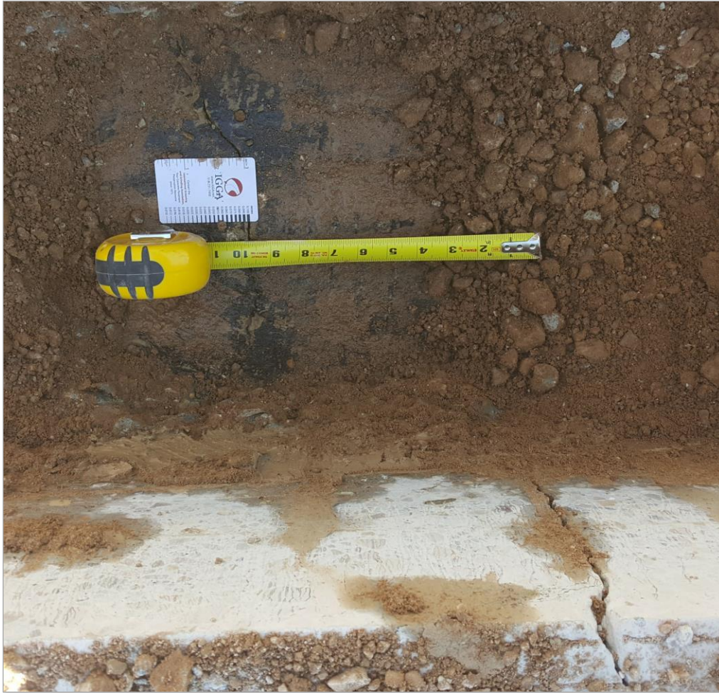
Figure 16: Soil cement base crack
