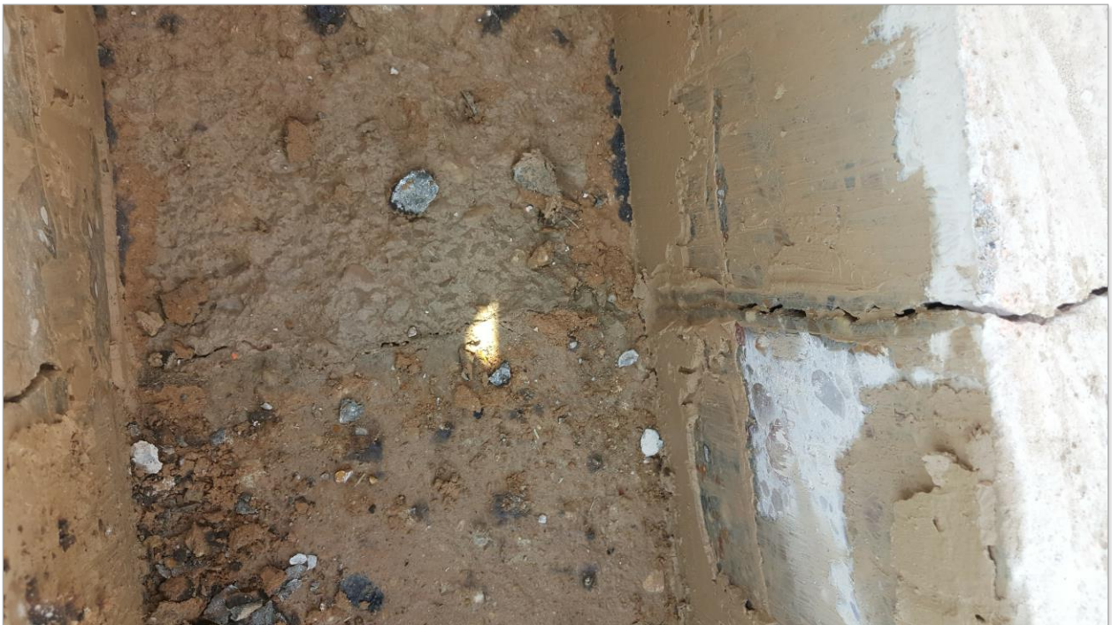
Figure 15: 4-inch granular crack
