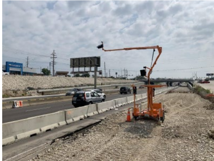
Figure 8: Trailer with Cameras and Sensor
