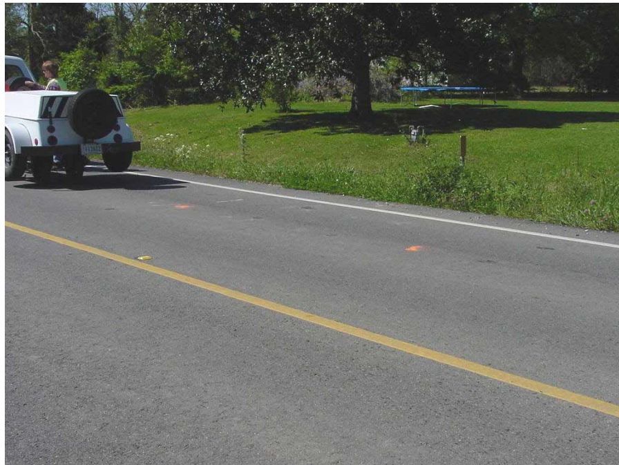
Figure 1-d. A Photo for the Problematic Cross-Drain Pipe Location on a Newly Constructed Highway
