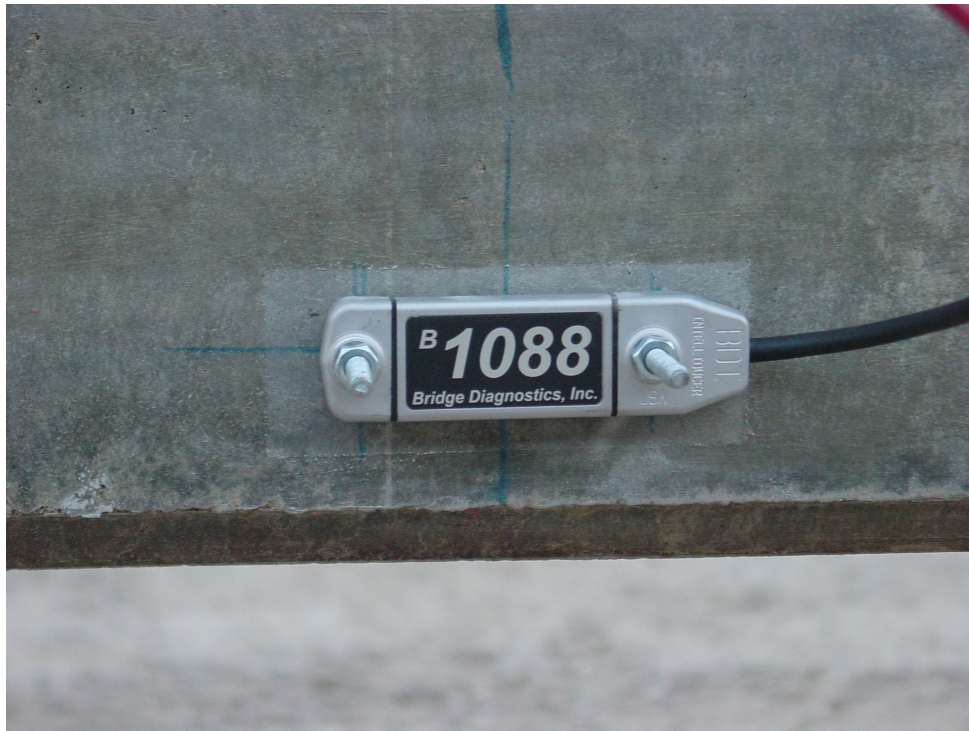
Figure 5 Installed strain transducer B1088.
