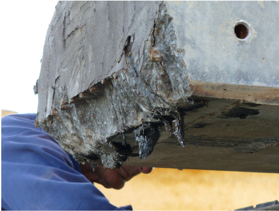
Figure 16 Beam B damage.
