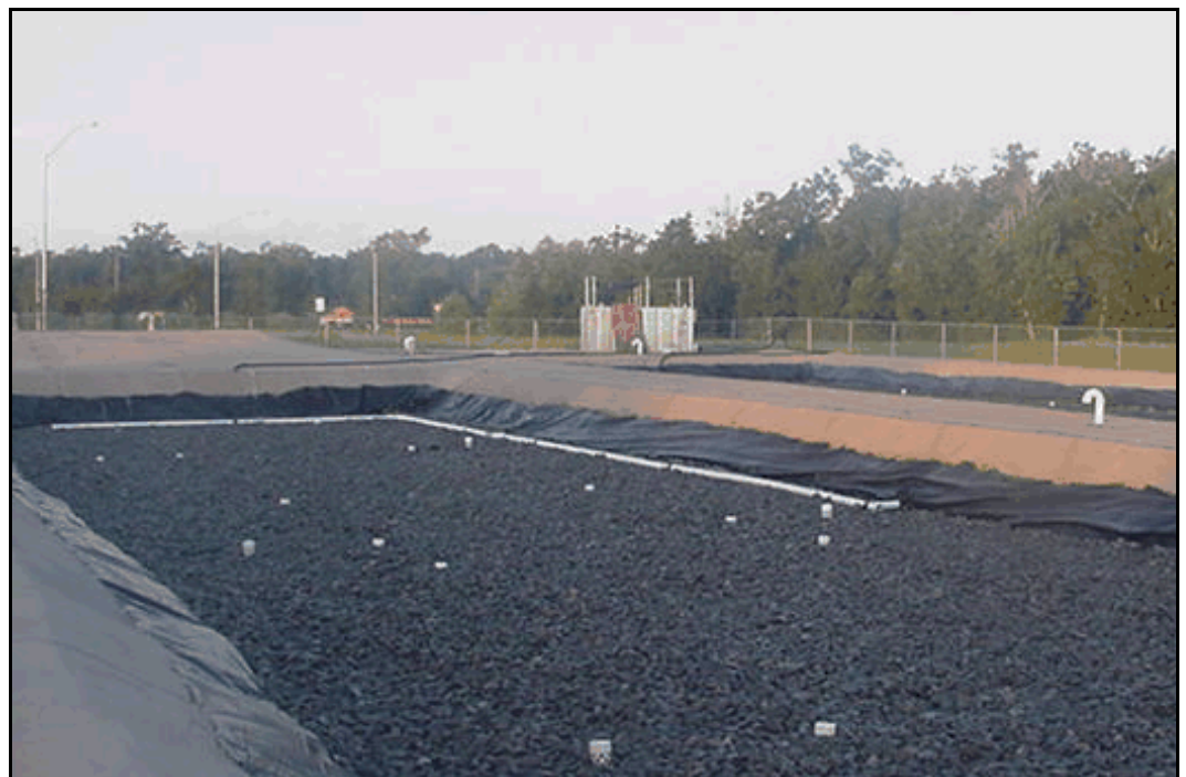
Rock plant filter (Grand Prairie SSF System)
