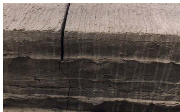
Development of controlled crack at the transverse joint.
