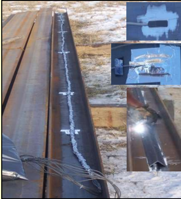
Steel H-Pile Instrumentation
