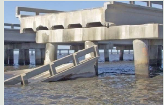
Figure 1 Interstate 10 damage following the passing of Hurricane Ivan
