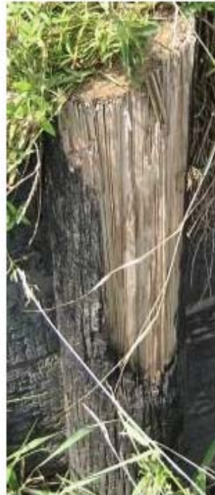
(c) Fire damage
