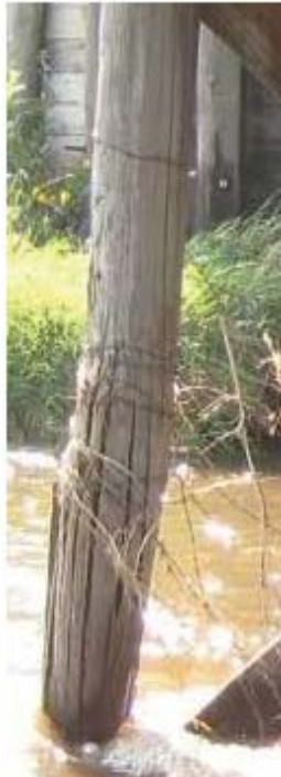
(b) Debris damage
