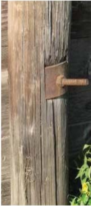
(a) Mechanical damage
