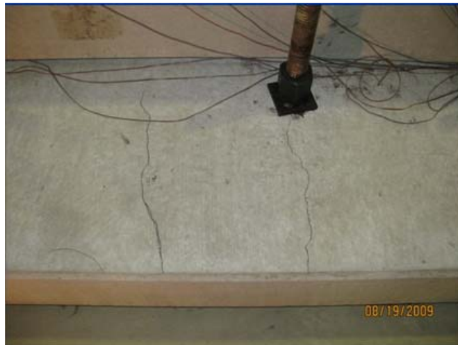
Figure 65 Cracks developing at top face of barrier slab
