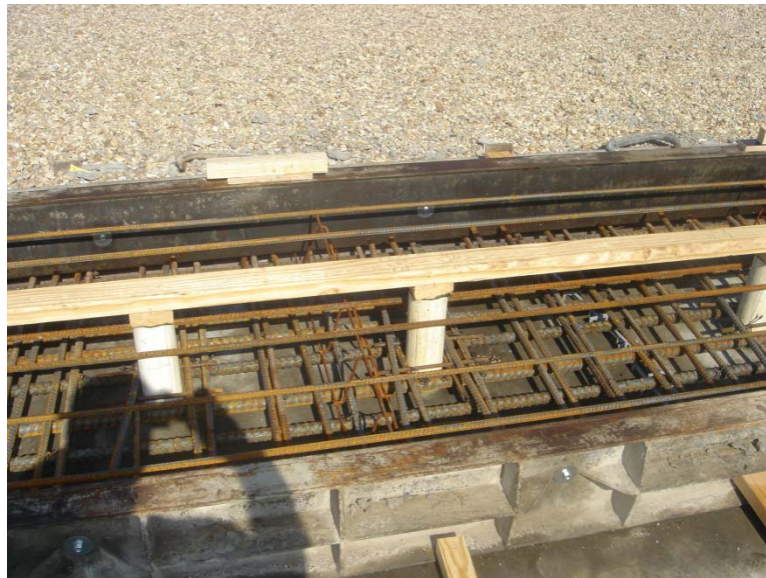
Figure 29 PVC Pipe blockings used for anchoring the slab to the strong floor
