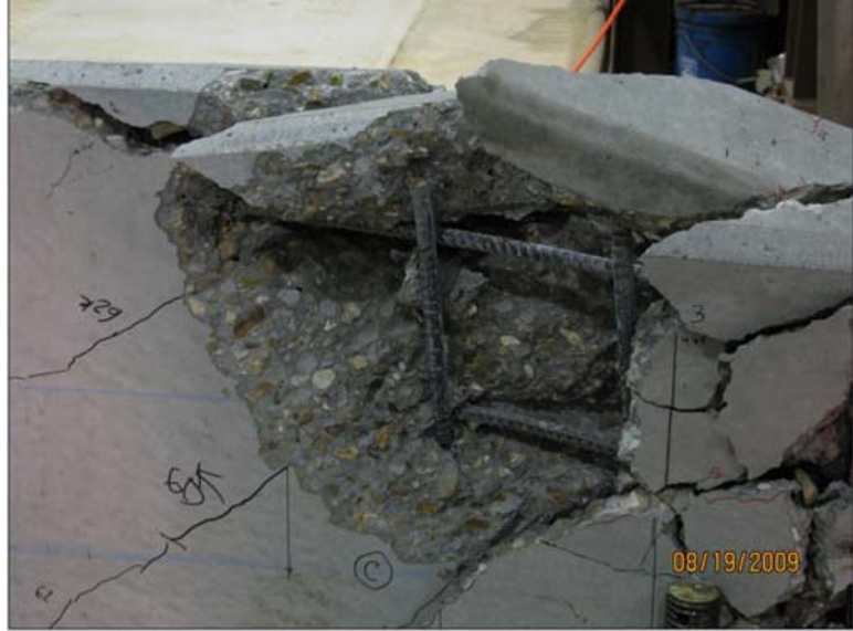
Figure 69 Close up failure at the top 11 in. of barrier (vertical face)
