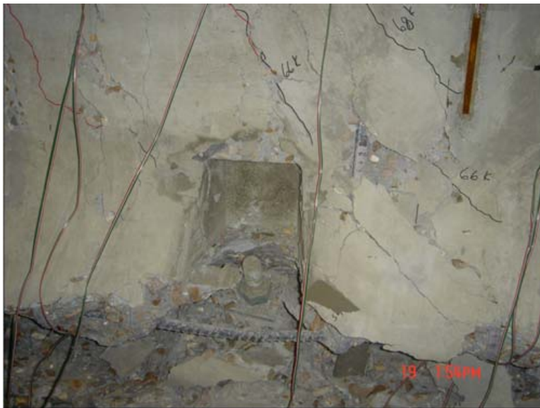
Figure 80 Close-up of breakout (notice intact anchor bolt)
