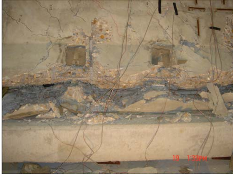
Figure 75 Failure of barrier at one of its ends (sloping face)
