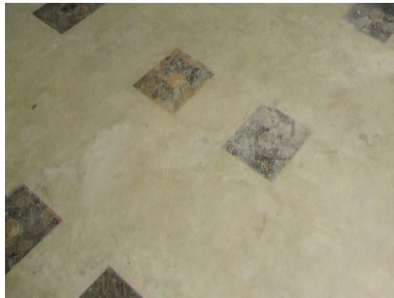
Figure 43 Black squares are heavy steel plates to protect threaded sleeves of anchor rods
