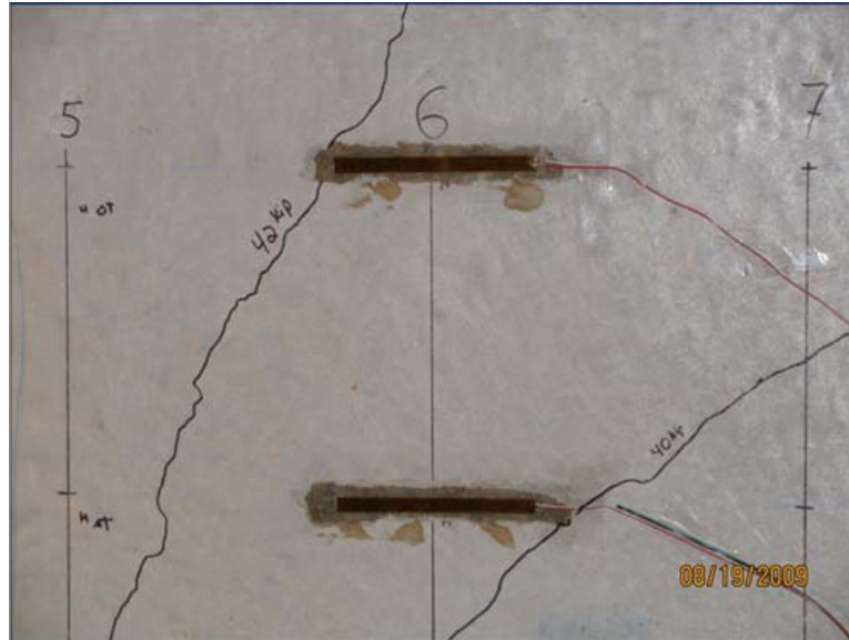
Figure 63 Diagonal cracks developing on vertical face of barrier
