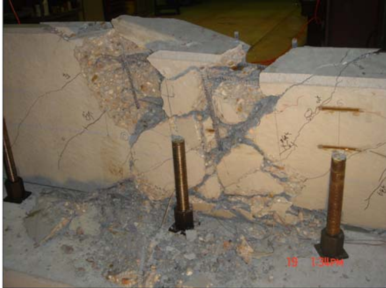
Figure 77 Torsional failure of barrier from vertical face
