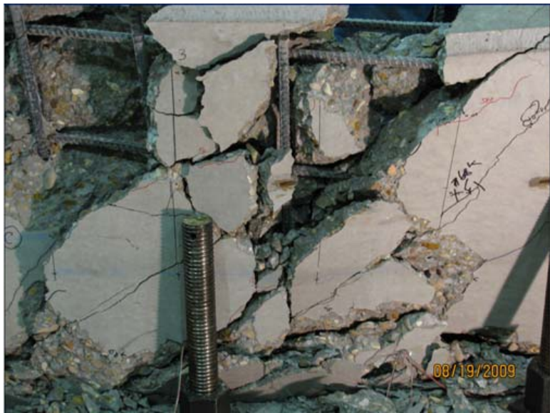
Figure 70 Close-up failure at bottom of barrier (vertical face)
