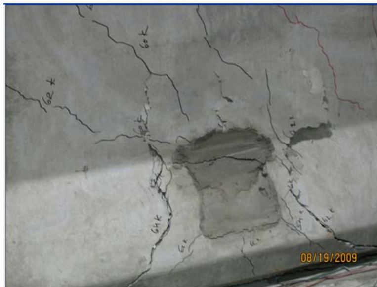
Figure 67 Diagonal cracks through barrier anchor supports
