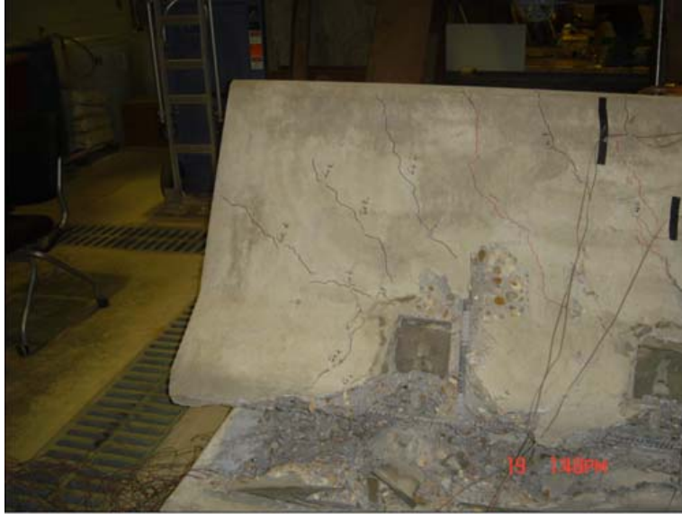
Figure 79 Breakout failure of barrier
