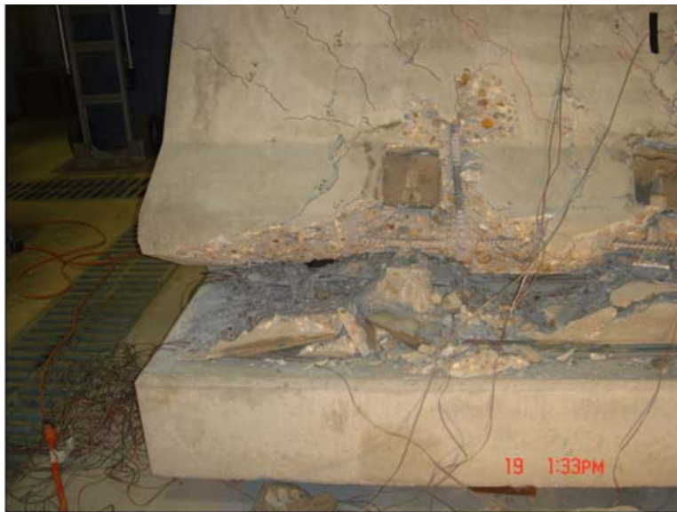
Figure 76 Close-up failure of barrier at one of its ends (sloping face)
