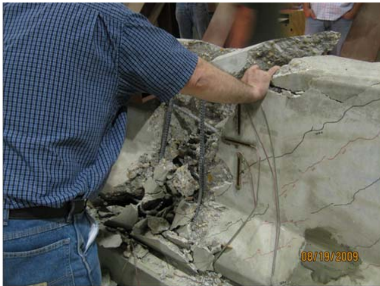
Figure 72 Cracked region of barrier (sloping face)
