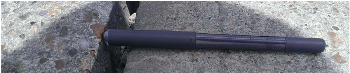
Figure 17 Faulting of adjacent pavement slabs for the 810-12 project slightly less than 1/4 in.
