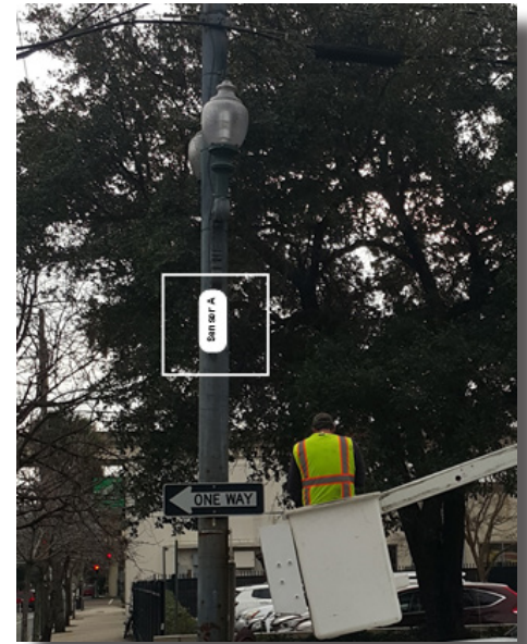
Figure 1 The mounting process of sensor A on a light pole
