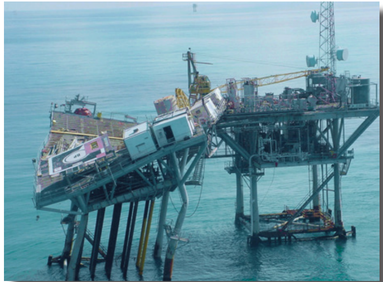
Figure 1 Damage caused by Hurricane Lili (2002)
