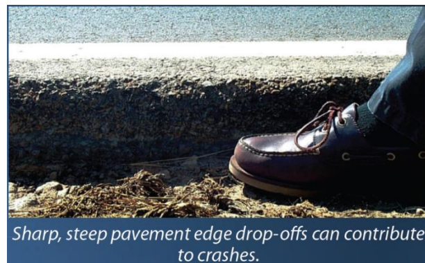
Figure 1. Extreme example of edge drop-off [2]
